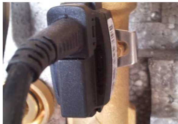
Fig. 8. Installed vortex flow meter
