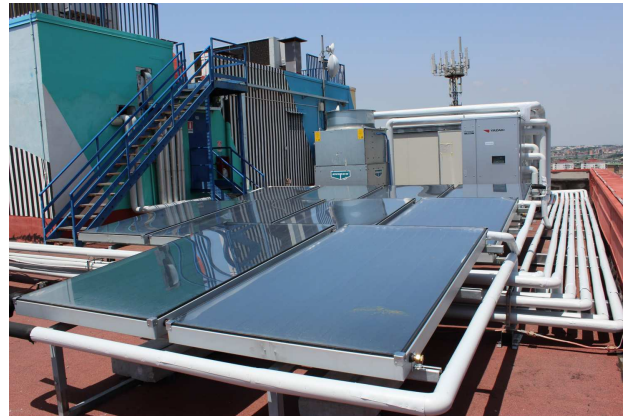
Fig. 1. A view of the SHC plant installed on the ABC headquarter roof
