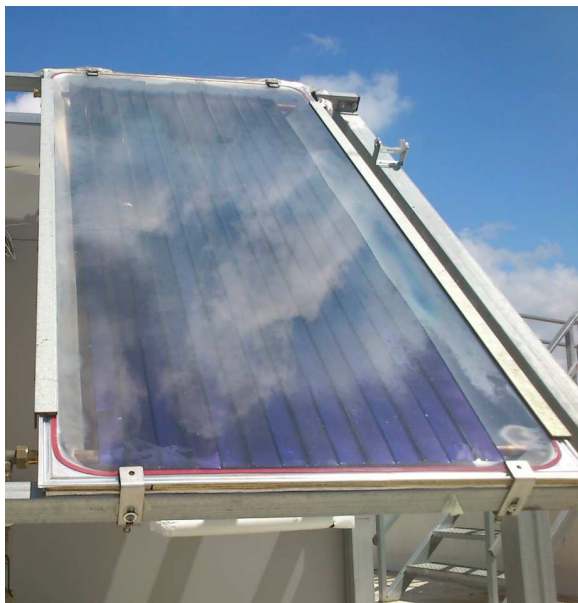
Fig. 4. Prototype of installed solar collector
